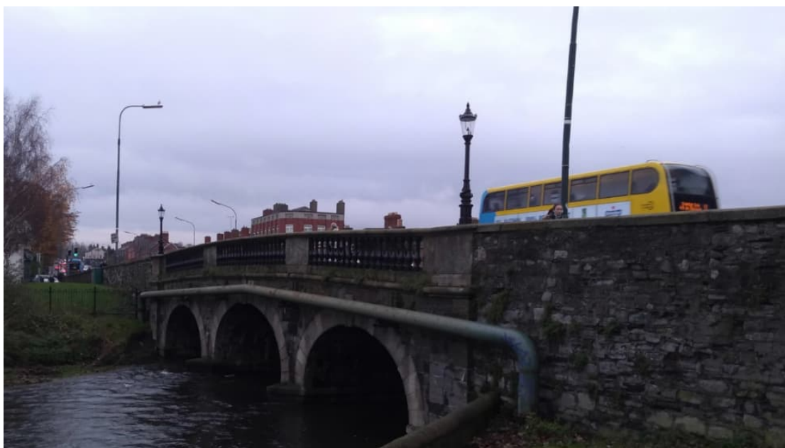
Figure 2.4: Image of west elevation showing large diameter gas main attached to spandrel wall
